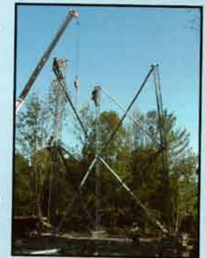
Construction is under way in Estill County, Kentucky, on a wireless broadband site for MCP's FEMA client that will provide communication for emergency services personnel in the protective action zone around the Blue Grass Army Depot. The project is part of the Chemical Stockpile Emergency Preparedness Program.
